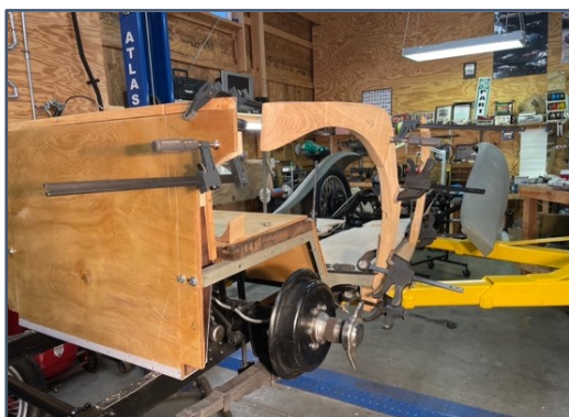
Rear tub showing the side curtain backing and wood frame and for the right quarter
